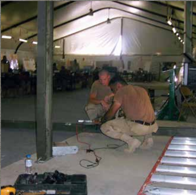
Construction of the large utility tent housing the Joint Operations Center (JOC) and other office spaces.
