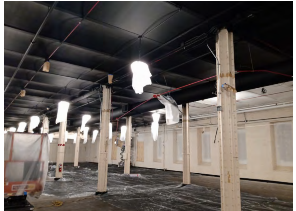
The Rock Islands Arsenal Museum is under construction for the installation of new galleries.
